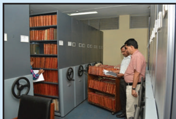
Shelving of back volume journals in newly installed Compactors at Dr. B.B. Dikshit Library
